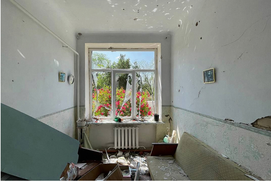
Fig. 11. Destroyed home in Mykolaiv region (photo: Serhii Belinskyi)
